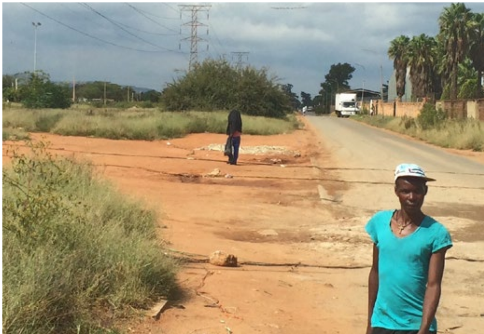
Illegal electricity connections running from Nancefield to the adjacent informal settlement
