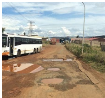
Potholes in Nancefield
